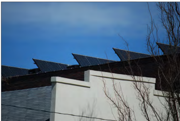
Solar collector panels are becoming increasingly affordable and are being developed in a variety of forms and scales, with this installation on a traditional apartment building.
